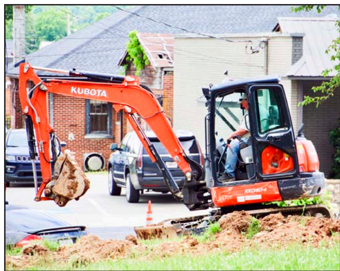
Hiawassee Water Department Manager Carl Grizzle working on a town square excavator to install new grizzuit on the Town Square Friday.
